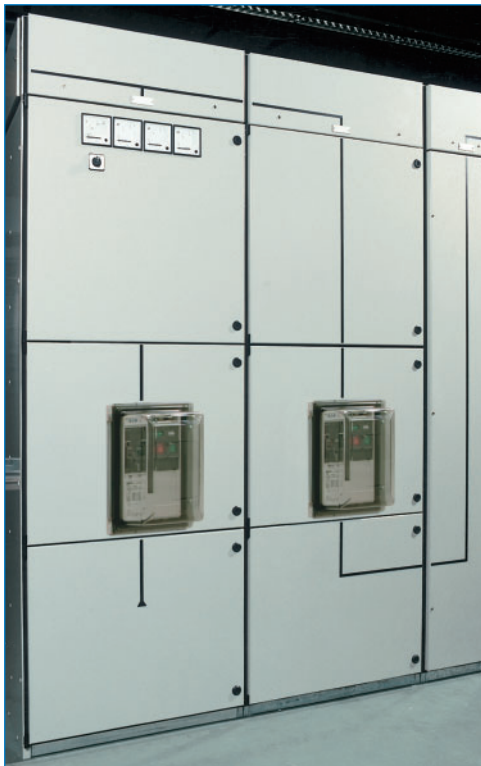
Capitole 40 assembly with Magnum Air Circuit Breakers as incoming feeder and buscoupler.
