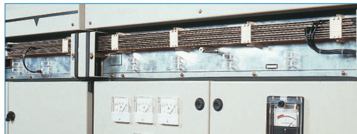
Auxiliary busbars in front of main busbar compartment.
