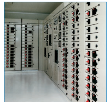
Assembly arrangement with corner cubicle.
